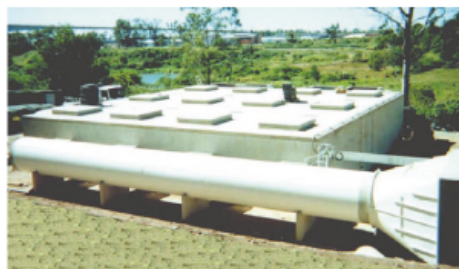
Clean TeQ ABOX system treating odours from rendering plant
